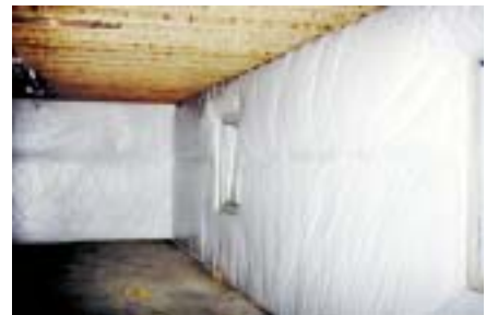
Photograph 3 Blanket insulation with impermeable vinyl interior surface
